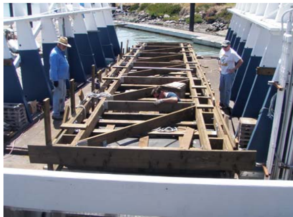
Mike Baldwin, Kim Arrivee and Keith Schardein prepare a new finger pier for A Dock
