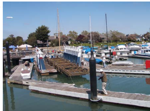
Mike Baldwin, Kim Arrivee and Gary McAfee push while Keith Schardein and Bob Frey control the first "splash" of the finger pier for A Dock
